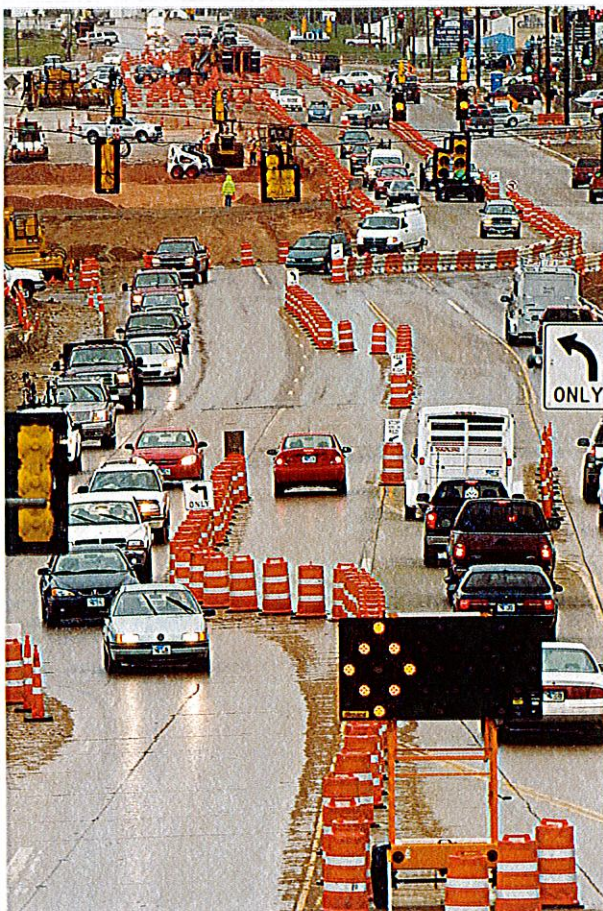
Construction continues on South Douglas Highway on Tuesday evening during rush hour. - News-Record photo by Sarah Voegele
